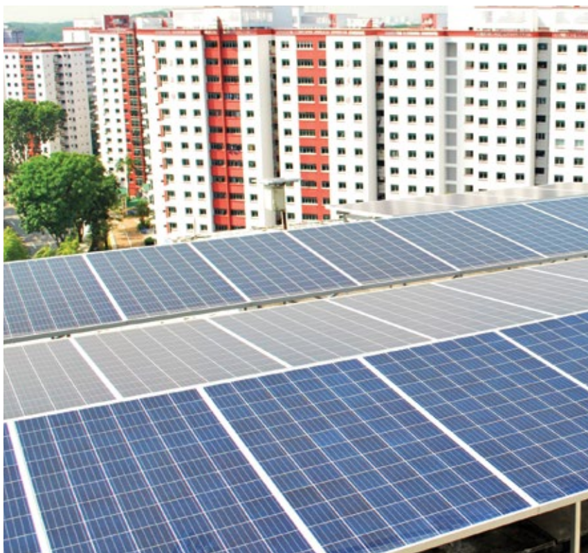
With close to 10,000 HDB blocks located islandwide, HDB is currently the largest driver for the installation of solar PV systems in Singapore. Image: HDB.
